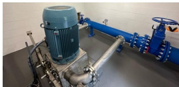
Figure 1: Community Hydro Scheme – Corwen Electricity Co-operative
